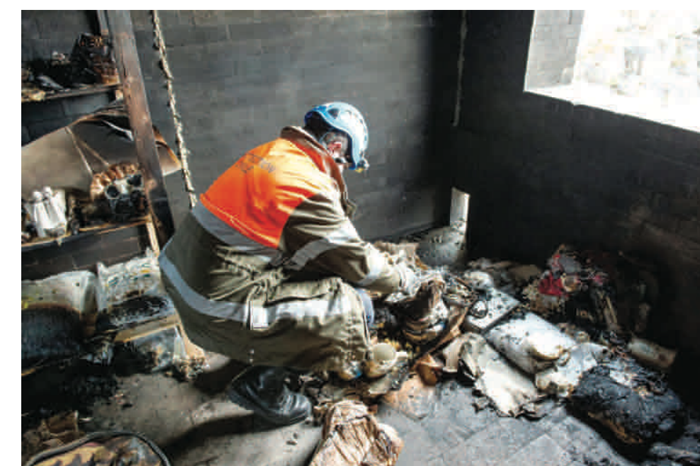
Fig. 6: A Civil Protection Agent preparing for the evacuation of objects from the disaster site. ©HE-Arc CR 2015
